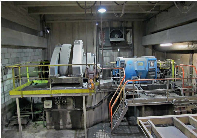
1 Gear unit in installed state prior to overhaul
